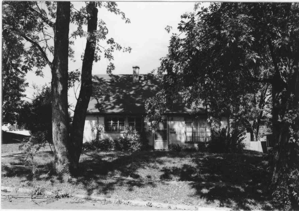
Oak Hills Subdivision: Photograph 10—Looking northwest at a house on Juniper Street within the Oak Hills 2 section. The house is a remaining intact dwelling, although it is deteriorated and condemned.
