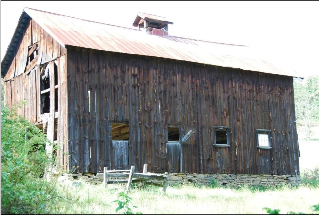
#802254—505 Christy Rd. Eighty Four, North Strabane Township, Washington County. A typical plain New England barn in a state of disrepair.
